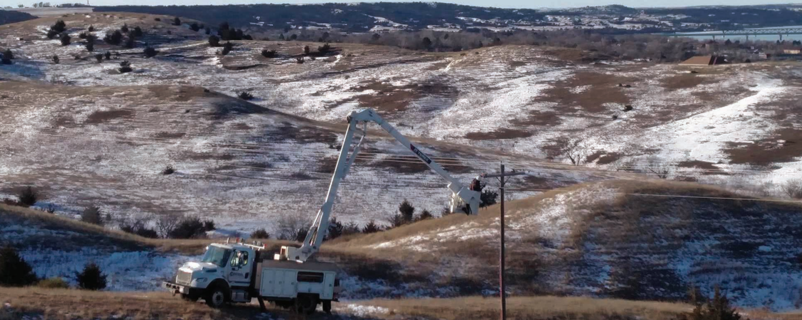
Lineman Jesse Baker repairs a “floater”, or line that became untied, north of Chamberlain following the storm. Photo taken by Lineman DuWayne Moore.
