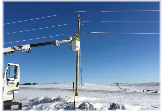
Lineman Jon Reichert repairs line near Ipswich, SD on FEM Electric's service territory. Photo by Lineman Norton Truman.
