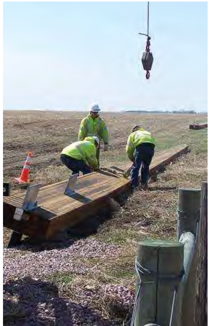
East River Electric crews building replacement transmission lines in Davison and Aurora County in 2014. The line provides electric service to the Plankinton Substation.
