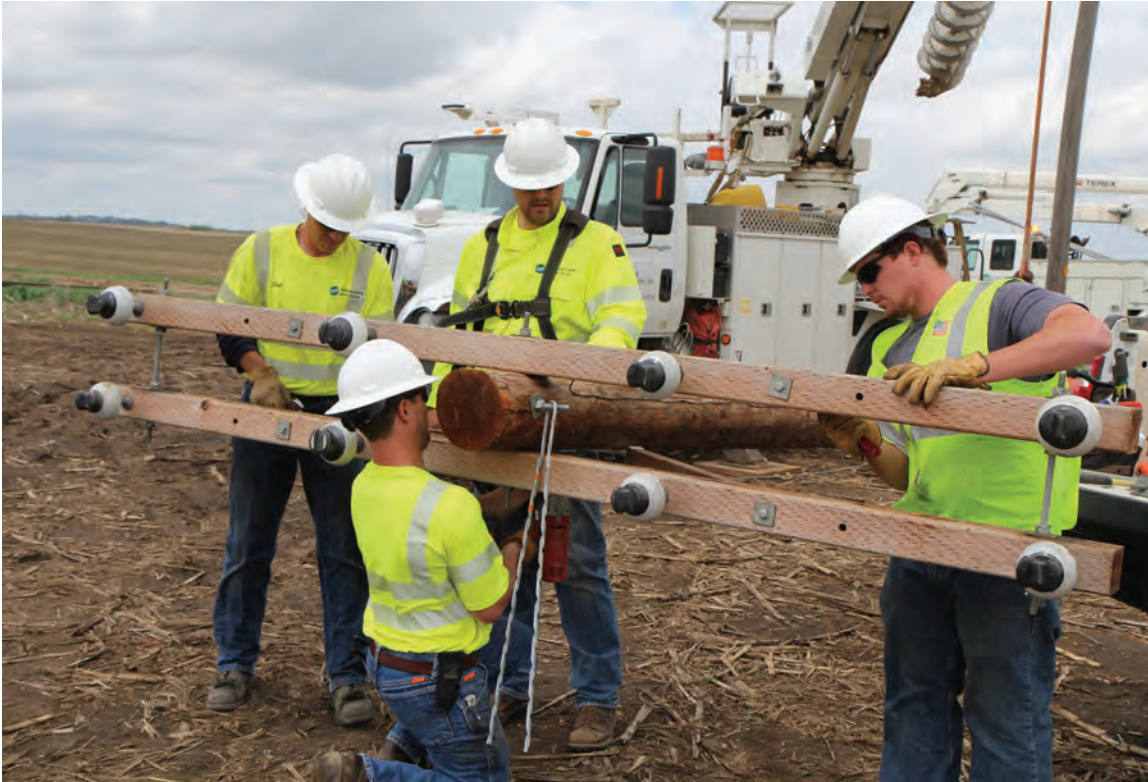
Left: 1,000 hour employee Nick Kramer, right assists a Codington-Clark Electric Cooperative crew with framing a pole for a pole change out south of Watertown in May 2013. Opposite Page: Kramer works on attaching a crossarm as part of the ground work he did during his 1,000 hour experience at Codington-Clark.
