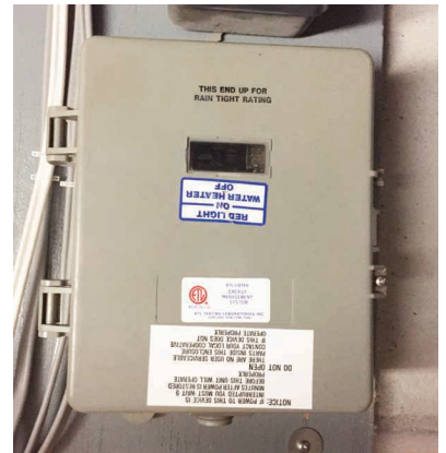
Above: These are the current load management boxes in most homes. These will be replaced.
