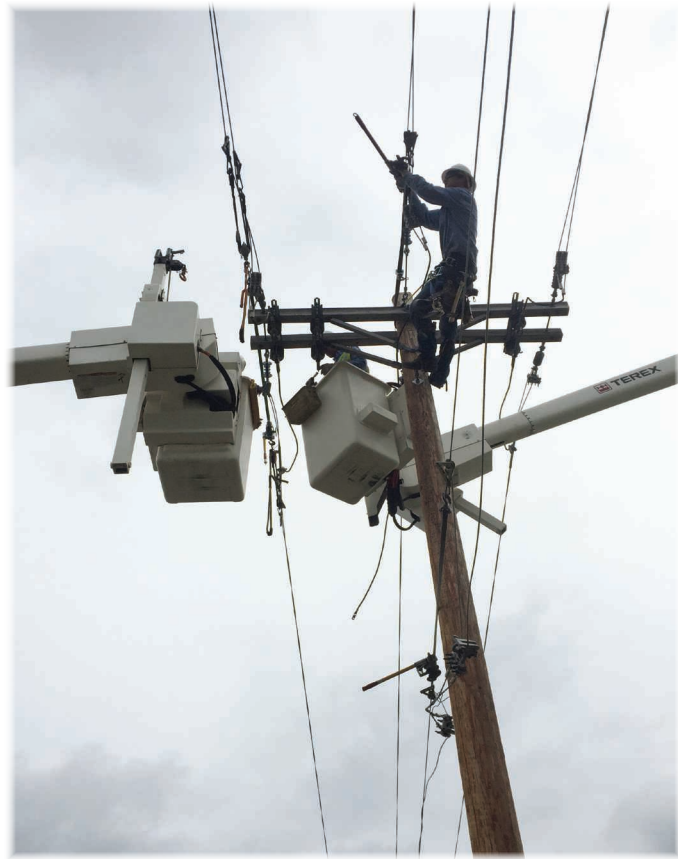
Crews perform a planned outage to replaced a burnt pole. Lineman Cody Riggs works on reattaching wires at the top of the new pole. Linemen John Vetch and Tony Roth assist nearby in the buckets.
