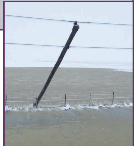
Additional barriers, such as standing water or deep snow, made repairs difficult.
