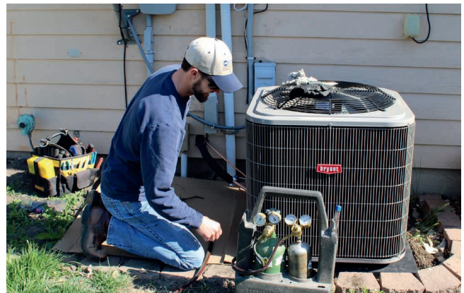
Aaron Punt and the rest of the HVAC team can install home heating and cooling systems. Ductless options are also available.
